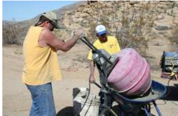
Above— Keith Walton mans the cement mixer, first making cement for patching, and then Merlex to water seal the rain apron. Below— Cement patch work needs to be smoothed to a fine finish before Merlexing.
