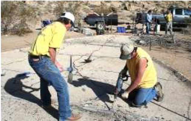
Above— First repair step is chipping away old tar patches from rain apron before new cement can be laid down to repair the apron. Below— Dave Smith and John Shaver repair fence and install walk-thru passage in fence.
